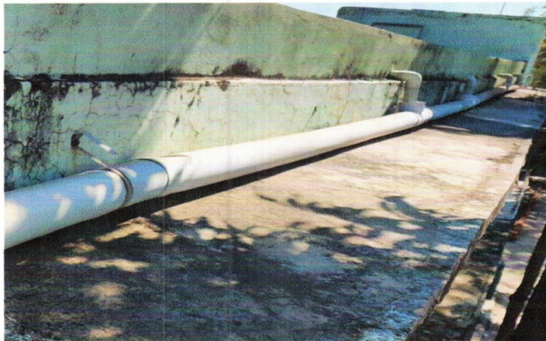
Photograph of Rain Water harvesting pipe
