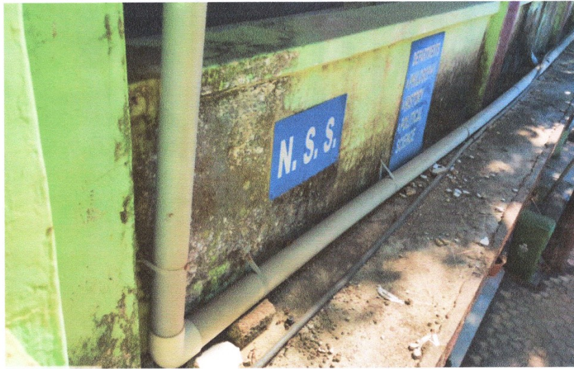
Photograph of Rain Water harvesting pipe
